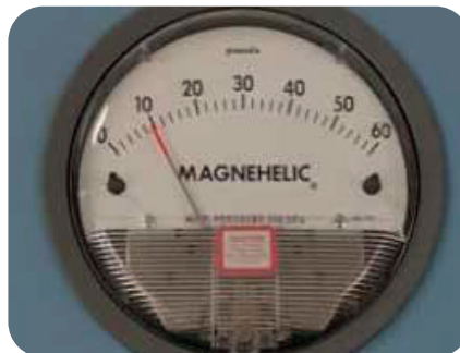
Magnehelic work chamber negative pressure gauge
